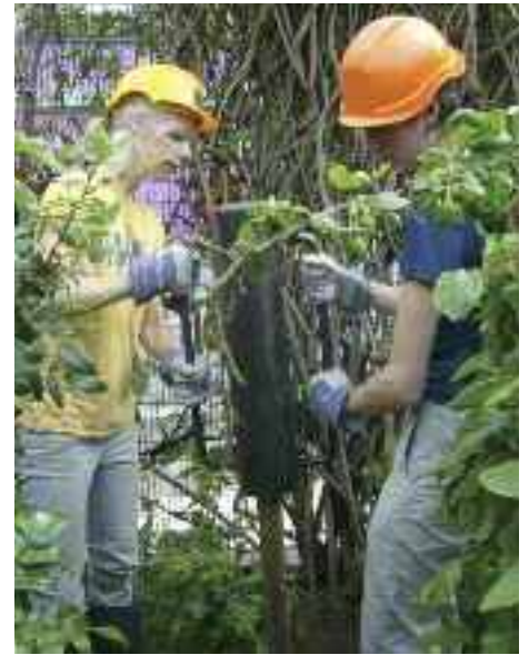
At Better Bankside, with so much property development underway, the BID has promoted a strategy for the spaces between buildings, looking for opportunities to steal space for incorporation in the public realm through carefully designed interventions. Making what little space there is available work harder, is being pursued through the introduction of containerised planting and placement of pink chairs
